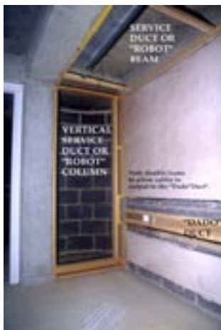
The interior of the 'Ark' building absorbs the concrete pillars and 'bressumers' into the folded walls and ceilings of the 'Working order' .
