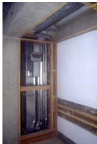
The hollow entablature of the Working order conducts horizontal M & E services between the pairs of concrete 'bressumers' that rest on the paired pillars.
