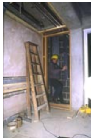
Two 300mm (1'0") sq concrete pillars and a 900mm (3'0") wide duct make up the 1.5M x 1.5M (5 ft. sq) body of the Working Order Column.
