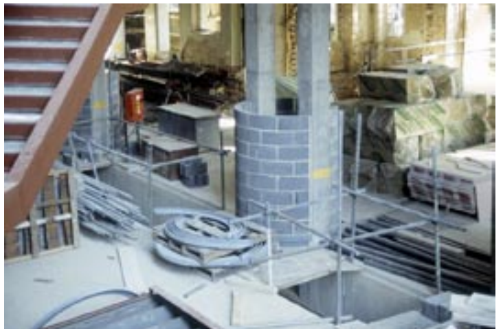
The feet of the 'necklace core' Gallery columns are connected by a tunnel in which run the drains, pipes and wires that then climb up to each floor.
